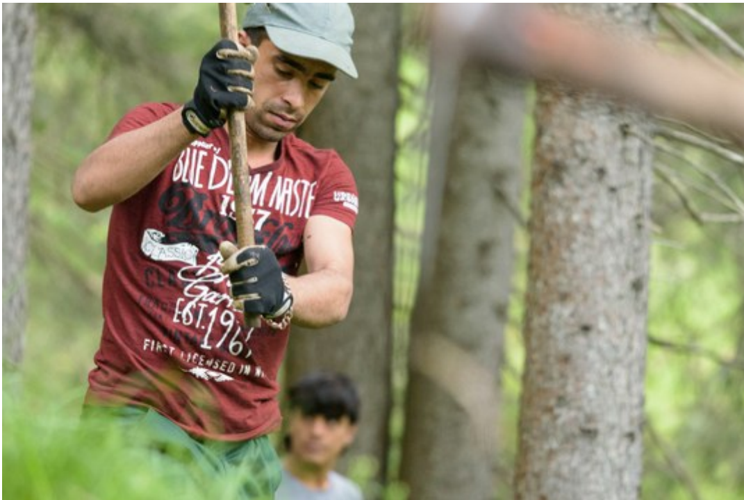
Construction of a steep path in the high mountains Copyright: Bergwaldprojekt e.V.
