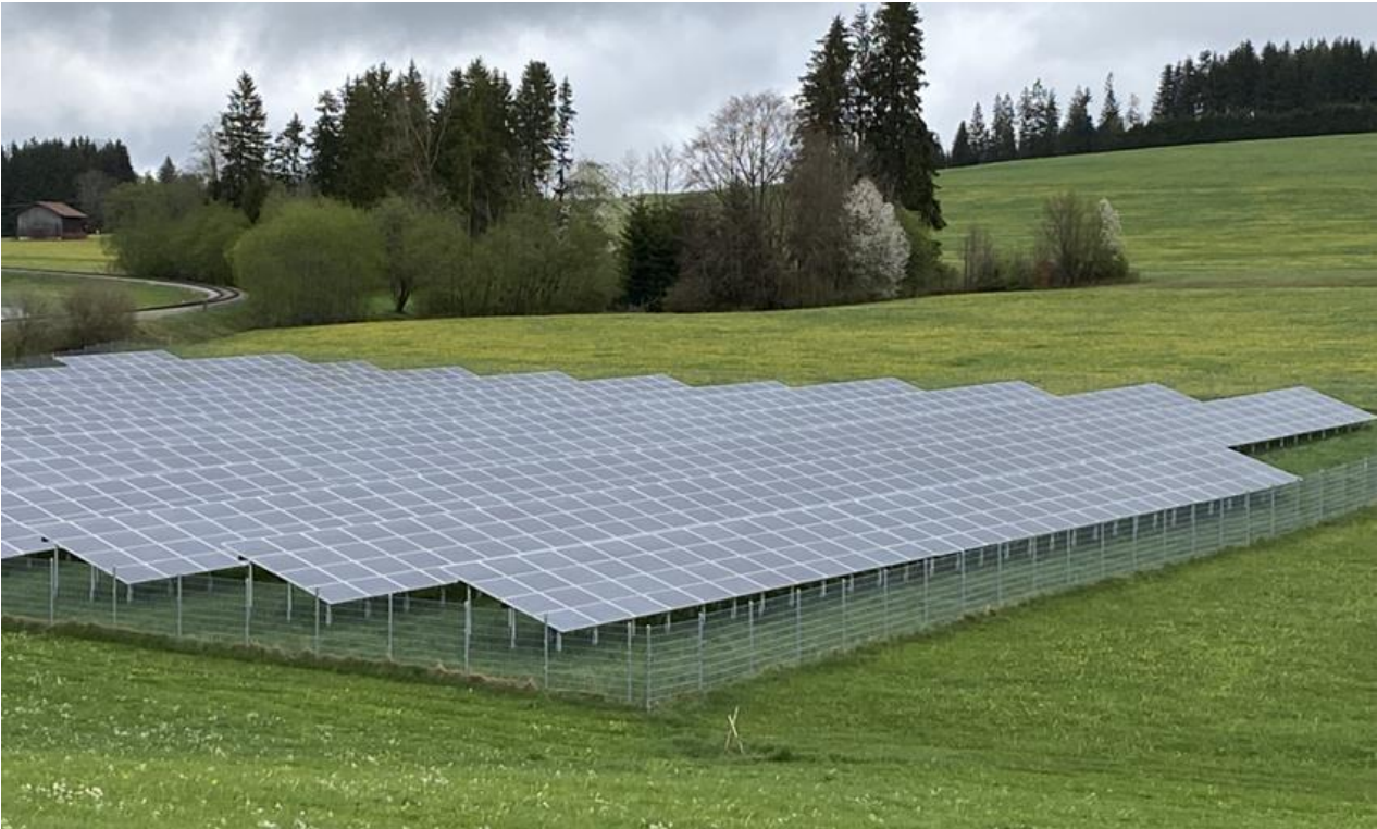
Figure 3: Ground-mounted solar panels
