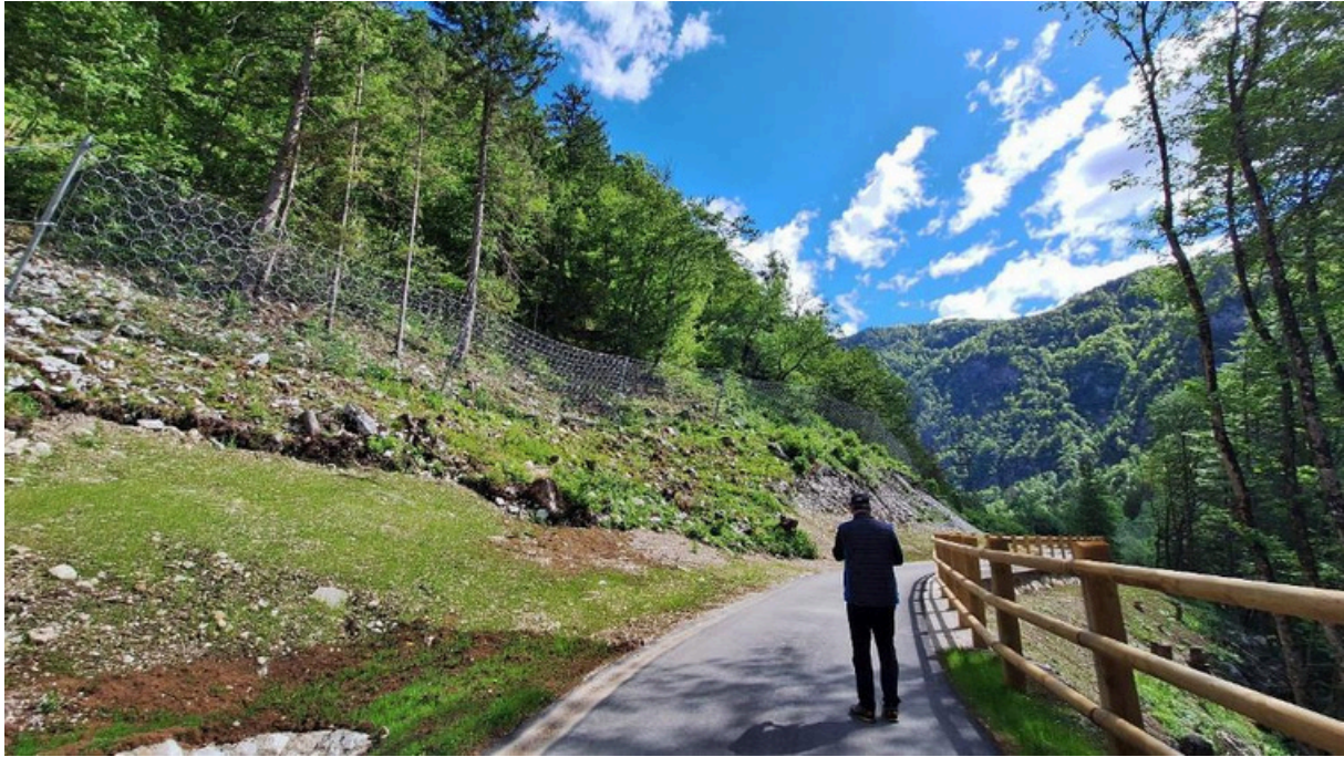
Figure 17: Rockfall protection barriers above the cycling path in Soteska, photo: Magdalena Cholkova
